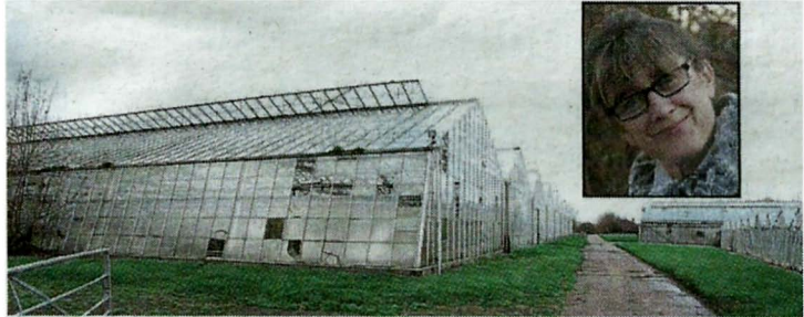
REDEVELOPMENT PLAN: Disused greenhouses in Great Horkesley, where homes could be built. Inset, Kate Charlton-Jones of the Stour Valley Action Group
